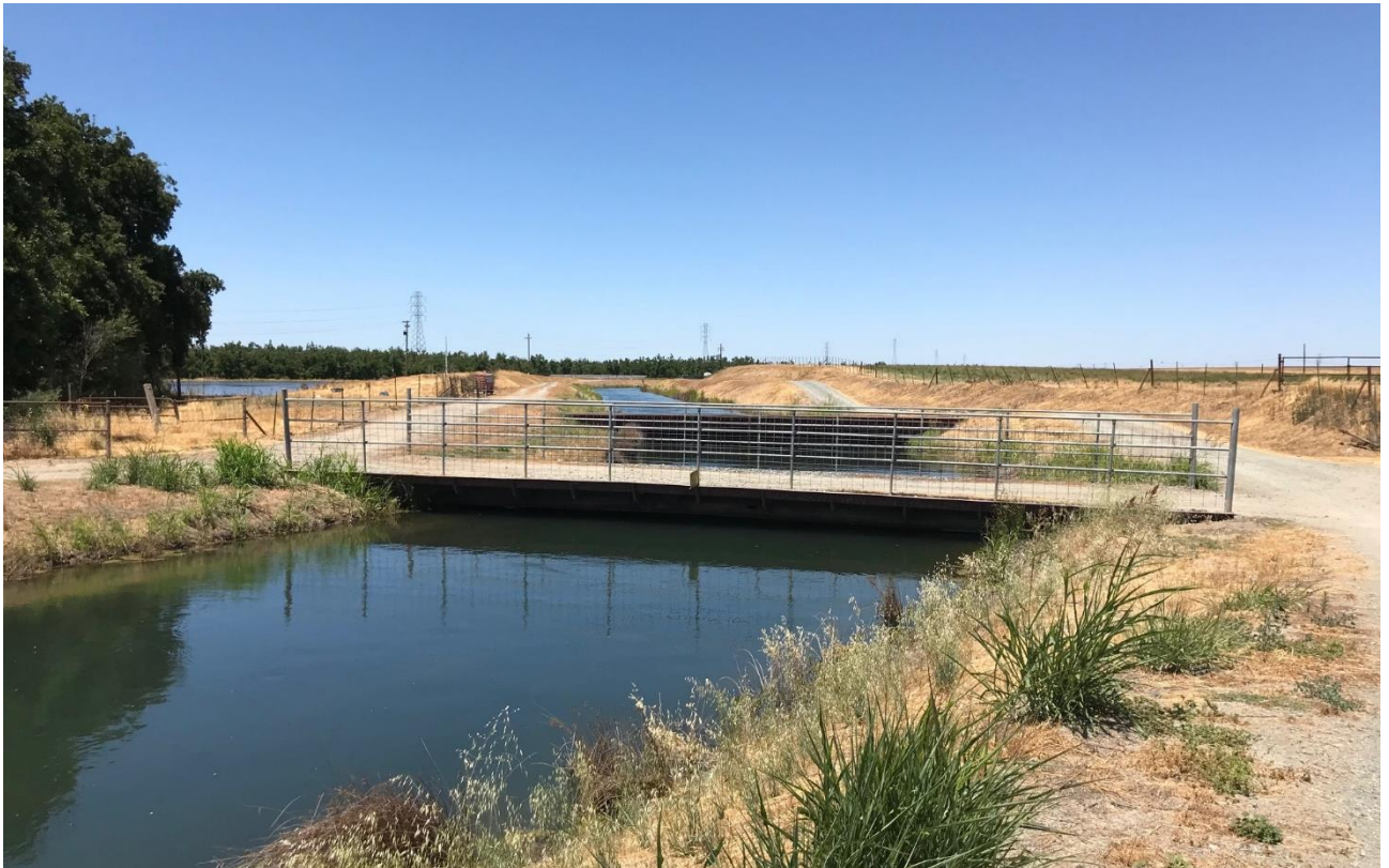
Figure 6. LFC Water Surface Elevation Reaching Van Vliet Bridge
