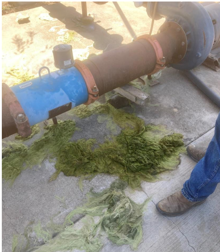
Figure 2. Vegetation Removed from Plugged Pump
