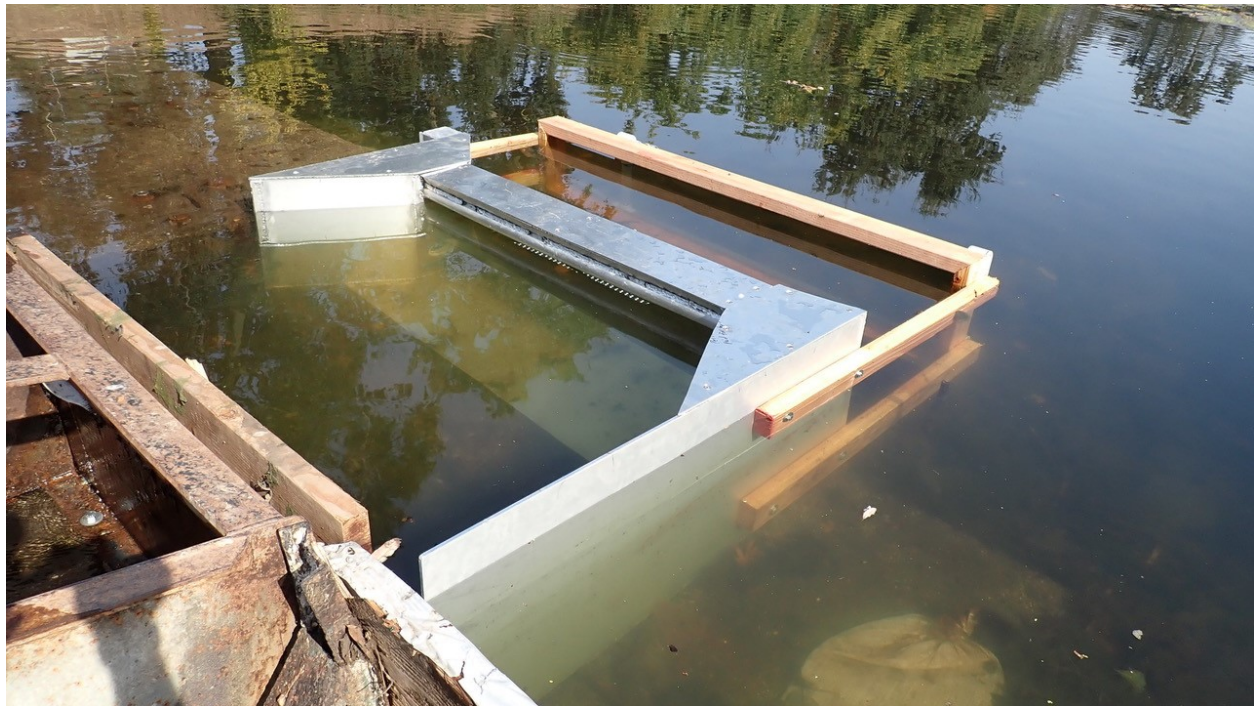
Figure 15. Above photo shows the custom passage chute extending into the upper pool. The chute serves to both extend the ladder to the upper pool while crowding passing fish near the internal cameras to ensure complete coverage.
